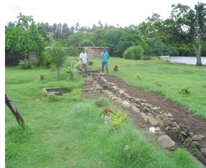
Above left: Native tree species seedlings supplied by the forestry department. Above: Drainage improvement project in Vanuaso village, Gau. The old drains were wider and more open.
